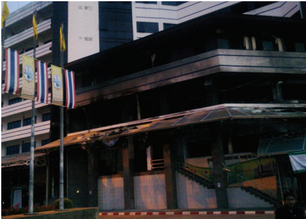
Façade of the Udon Thani city municipal office showing extensive fire damage caused by protestors who attacked and burned the front entryway, and bottom two floors of the building on May 19, 2010. © 2010 Human Rights Watch
