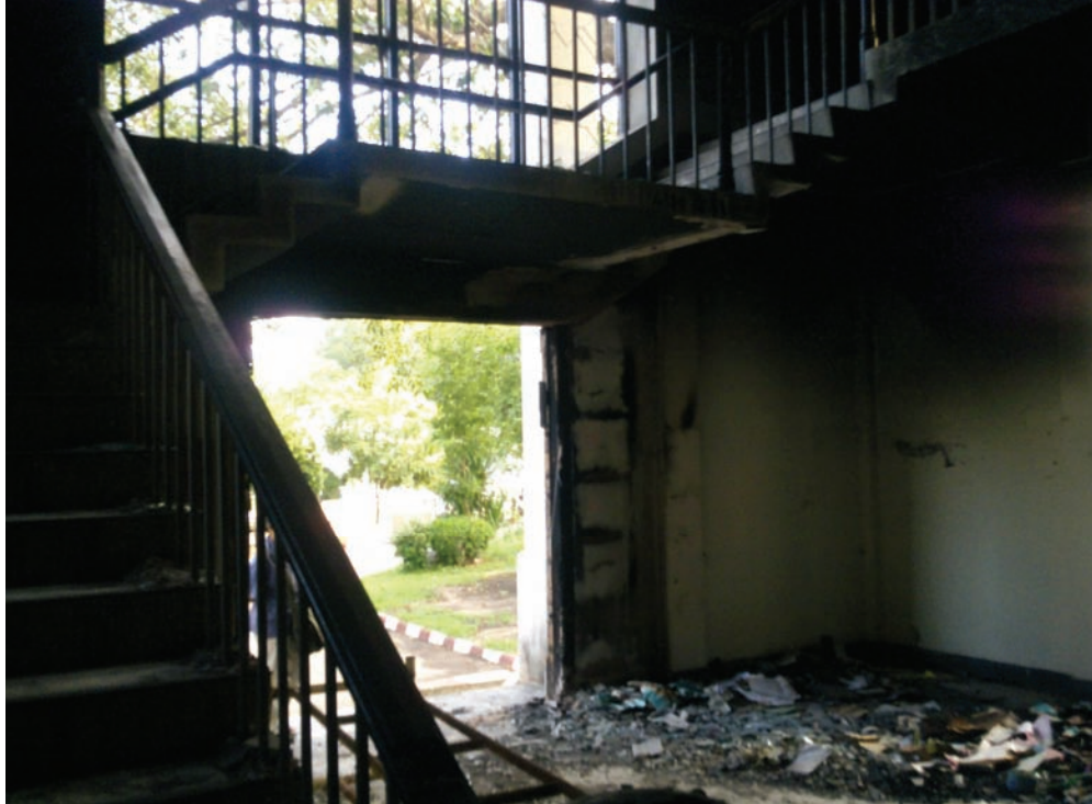
Burned-out side staircase on the ground floor of the Khon Kaen provincial hall, damaged by protesters on May 19, 2010. © 2010 Human Rights Watch
