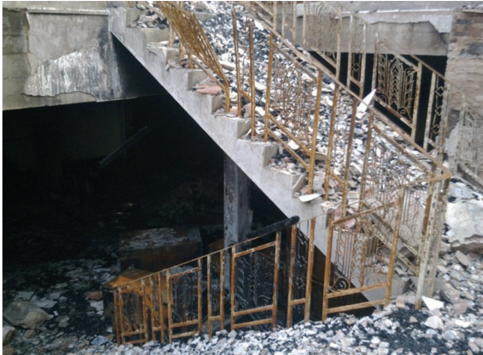
Rubble and fire damage on third floor of central staircase of the old wing of the Khon Kaen provincial hall, showing the destruction caused when it was torched by protesters on May 19, 2010. © 2010 Human Rights Watch
